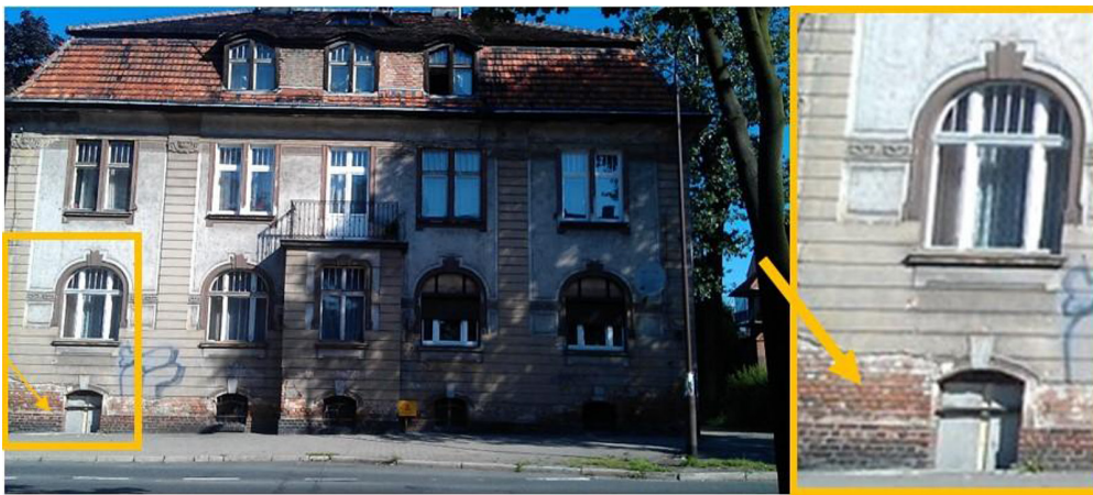
Fig. 2. Lack of horizontal and vertical insulation and degradation of old drainage systems, Jelenia Góra, Wojska Polskiego Av.
