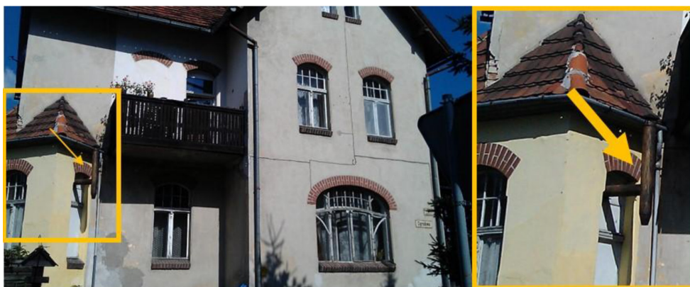
Fig. 4. Unauthorized construction work – chimney sticking out of the window after installing heating, Jelenia Góra, Ogrodowa St. Source: own photography.
