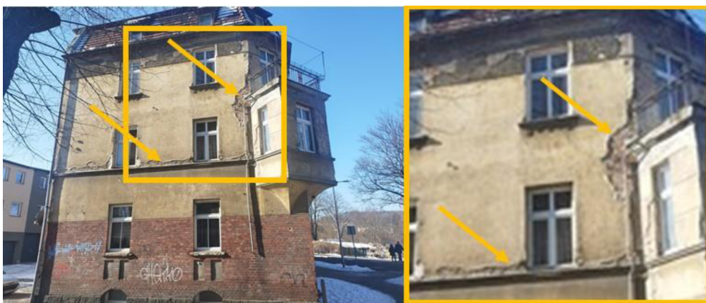
Fig. 3. Lack of horizontal and vertical insulation and degradation of old drainage systems, Jelenia Góra, Kasprowicza St.
