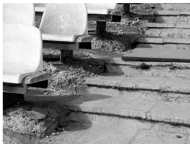
Fig. 4. Unsatisfactory condition of the tribune covers unsatisfactory condition of the tribune cover Source: created by authors (2021).
